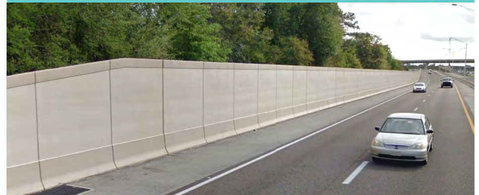
Example shoulder-mounted noise wall
